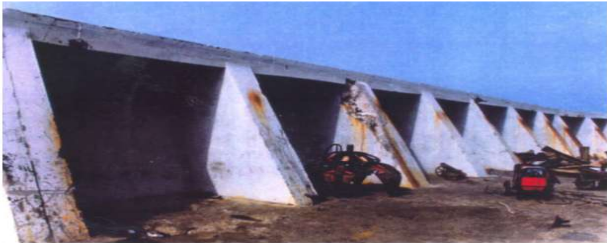
Figure 1.1: Corrosion of reinforcement by chloride attack in a marine environment (Walraven, 2008)
